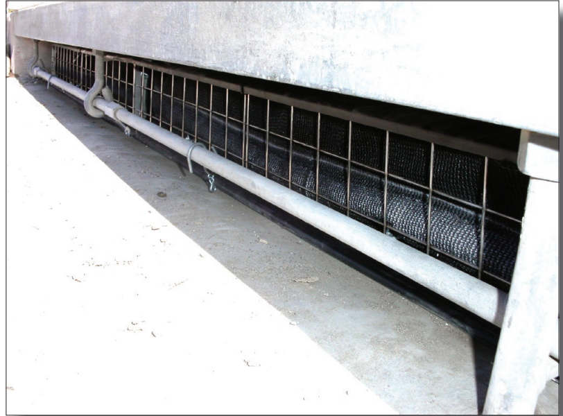
MODEL CP8 - INSTALLED
