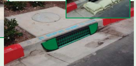
Curb Inlet Protection: Replace sand bags with re-usable protection!
